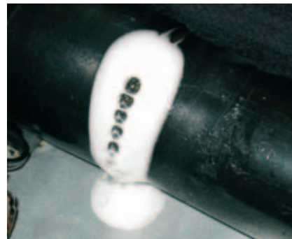
The leak is visible for several minutes.
