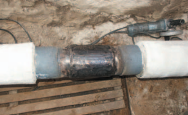
1. Pipe preparation as per GW 15, clean, dry and free of grease. If shrink sleeves are used, preheat to 70°C.
